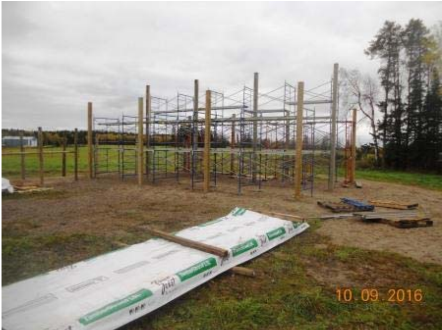
Photo: Construction begins with the framing of the caribou base facility barn.
