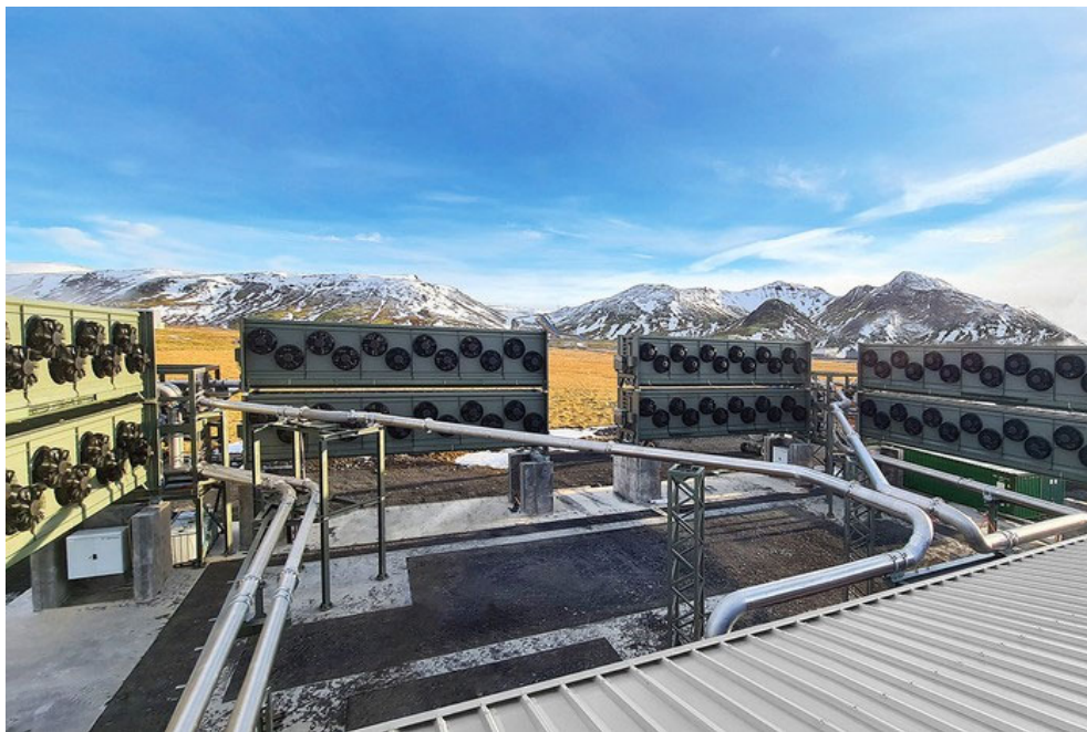
Figure 32. Orca Direct Air Capture Facility in Hellisheiði, Iceland 31
